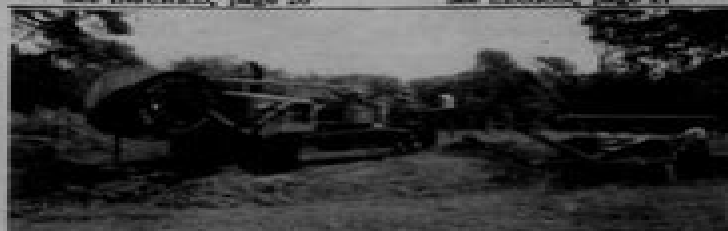
LAYING CABLE -- Trail - end cables between Lexington and Giddings are coming closer to reality every day as General Telephone crews lay a 200 pair cable along Highway 11.
